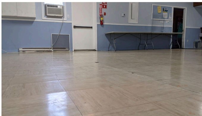
Photo 8: Uneven Floor Indicating Floor Joist Damage
