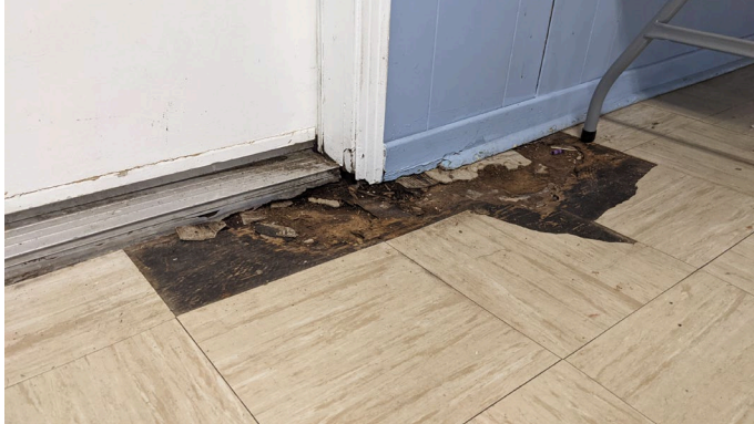
Photo 7: Courtyard Door Water Infiltration
