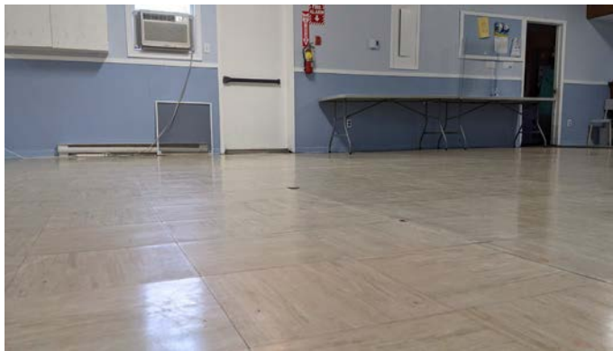
Photo 8: Uneven Floor Indicating Floor Joist Damage
