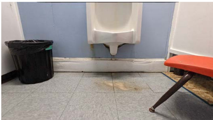
Photo 9: Male Washroom Floor Damage
