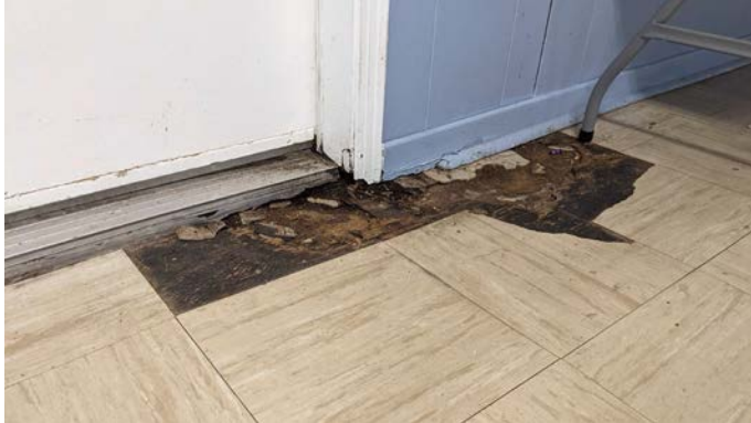
Photo 7: Courtyard Door Water Infiltration
